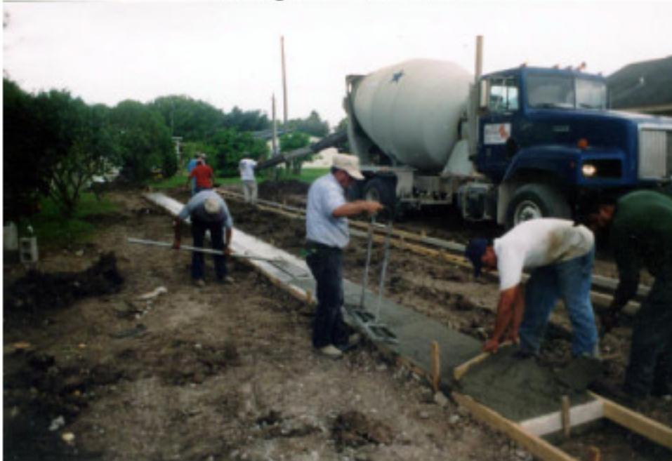
Pouring new concrete runners for new home. As these home owners had designed to have either a driveway, patio, garage, parking area, or sidewalk around and next to the entire home; they selected a foundation of runners to support their home and have the concrete around their home extend back under for their skirting. This saved money.
