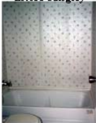
No protection for shower wall
