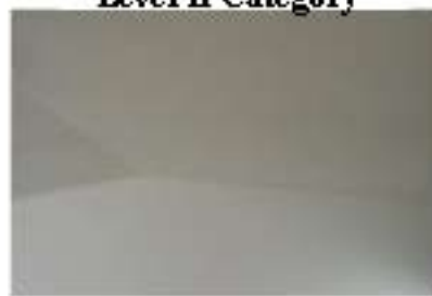
Blown Sheetrock Ceiling
